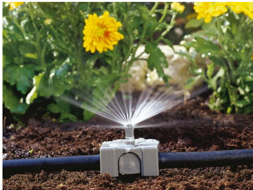
Figure 18. Automated irrigation. Source: verdeesvida
