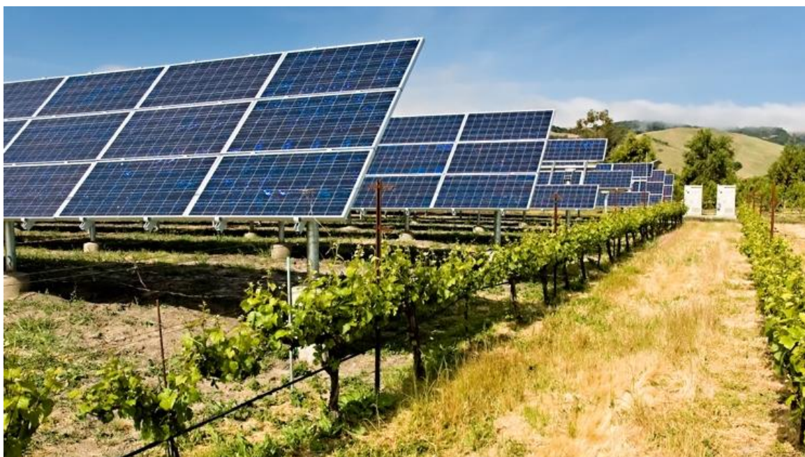
Figure 16. Agrivoltaics. Source: Iberdrola
